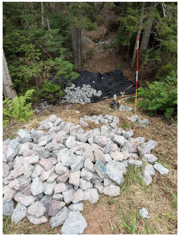
Figure 27. The early stages of a riparian bank stabilization project. Intended to capture runoff and filter water
