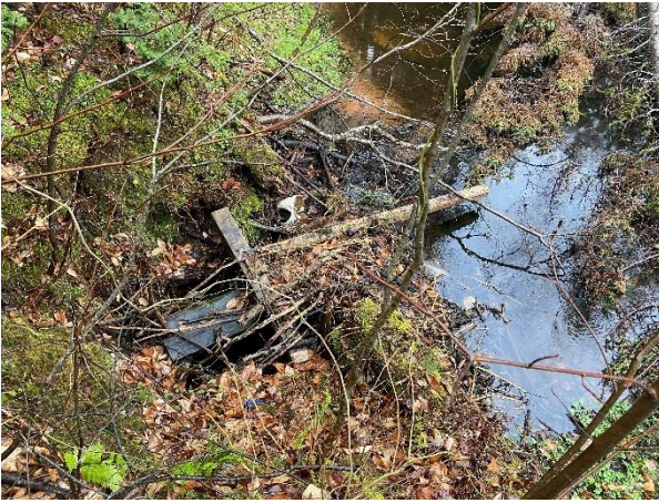
Figure 26. The discharge culvert is degraded and filled with debris and garbage
